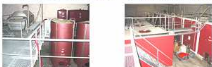
The catwalk around the pneumatic press.
